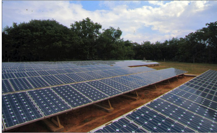
Fig 12. Photovoltaic Panel Array
