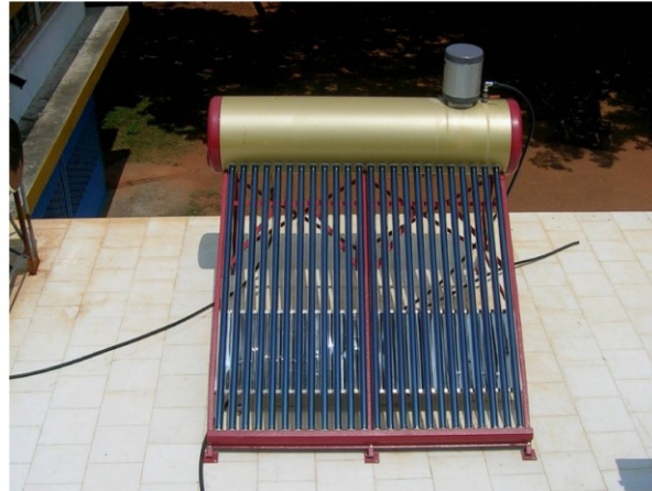
Fig 11. Solar Water Heater used in Auroville
