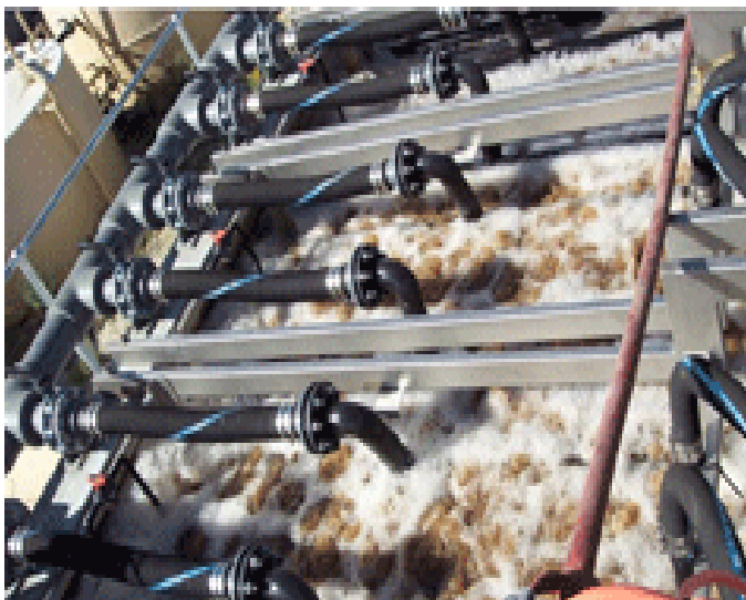
Image 7: Submerged MBR module during operation, Koch Membrane Systems, Puron[4]
