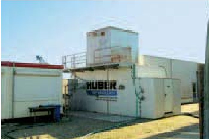
Image 8: MBR plant in container, Fa. Huber, Germany [6]
