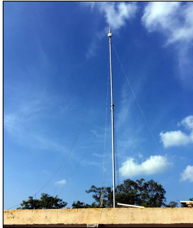
Figure 3—6 LoRaWAN antenna with receiving base station (gateway) installed on the roof of main CSR building
