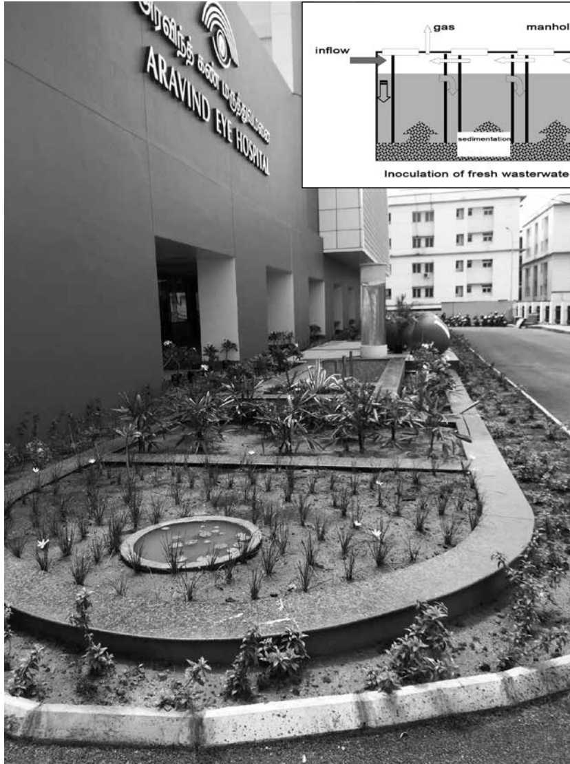
Waste water treatment plant installed by Auroville for the Aravind Eye Hospital in Chennai
