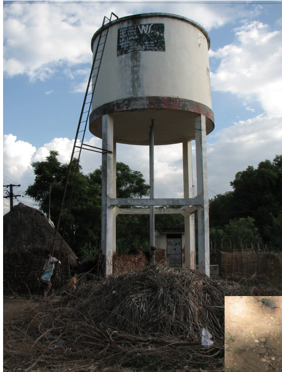
Elevated storage reservoir in Kottakarai
